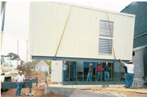
A Pre-Manufactured Distribution Center is transferred from semi trailer to its final resting place.
